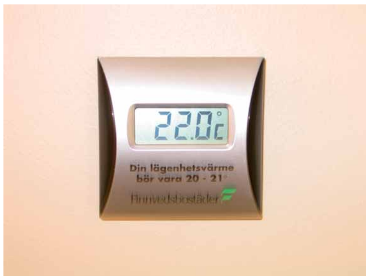
Figure 3.3 Display showing the temperature in each apartment.
