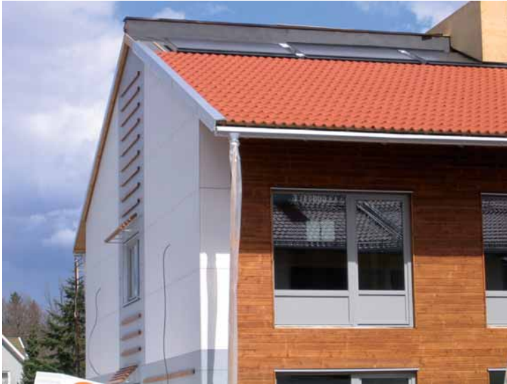
Figure 2.4 Solar collectors on the roof
