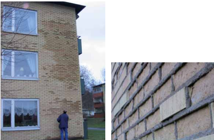
Figure 2.15 Worn out brick façade in Brogården
